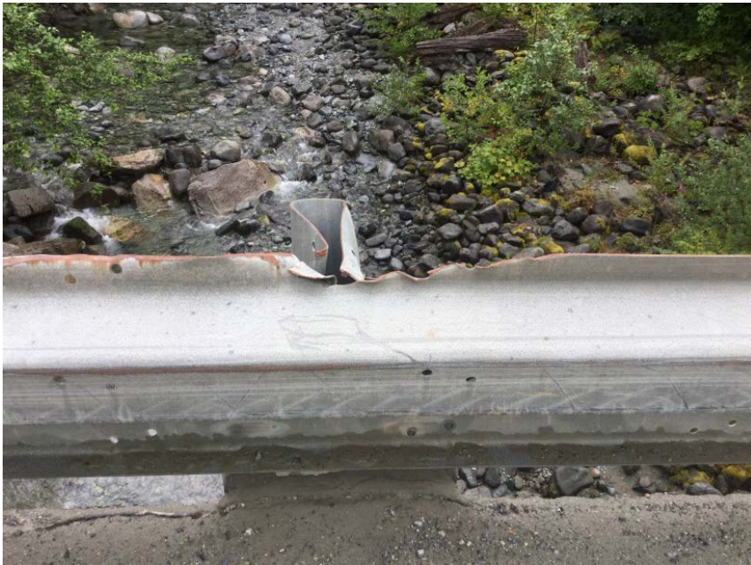
Damaged section of guardrail - still functional
