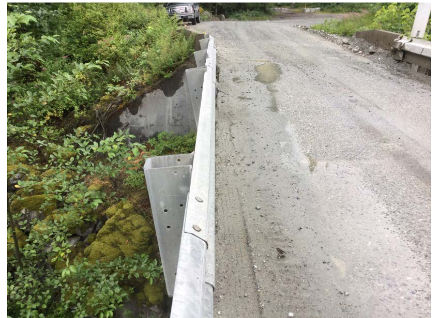
Guardrail damage downstream right approach - still functional
