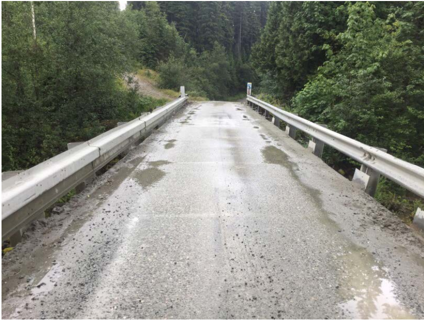
Different style of W beam rail upstream vs downstream
