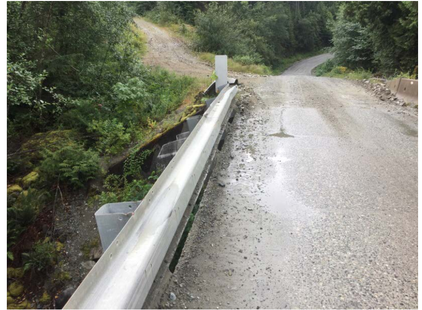
Guardrail damage upstream left approach - still functional
